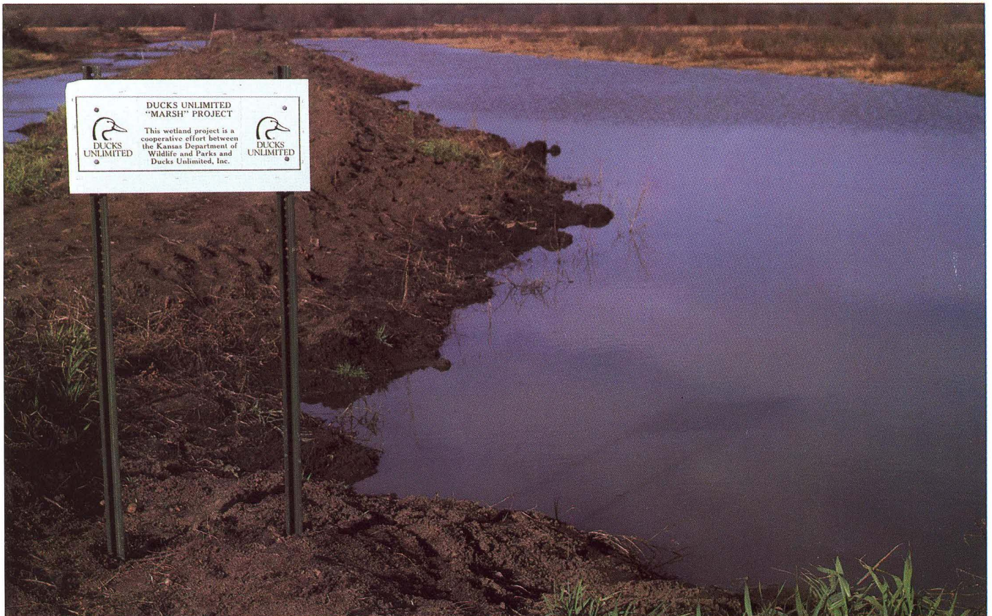
The matching money provided through Ducks Unlimited's MARSH program pays for acquisition of new wetlands and projects on existing wetlands. The construction of this dike will create more valuable acres of wetland habitat.
